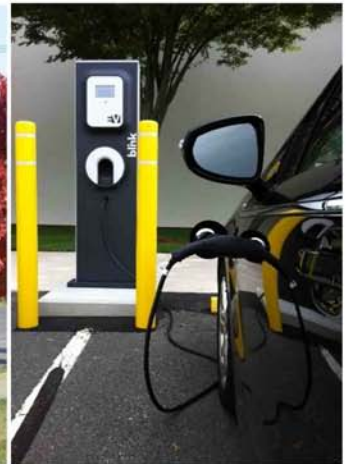
EV CHARGING STATION
